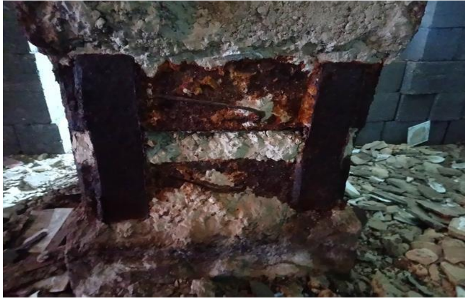
Figure 2. Exposed, highly corroded joints of the Column interface (along the axes 6-B, 6-C, 6-D, 5-D, 4-D) are in a pre-emergency state
